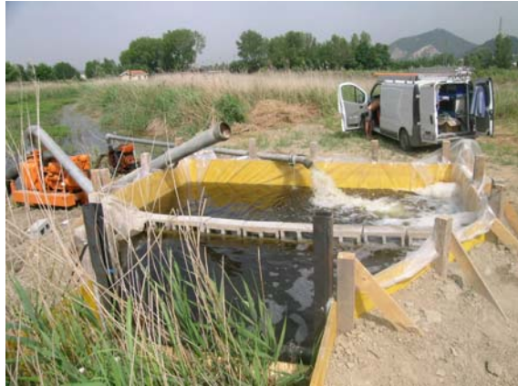
Figure 2: Water pumping into the head tank.
